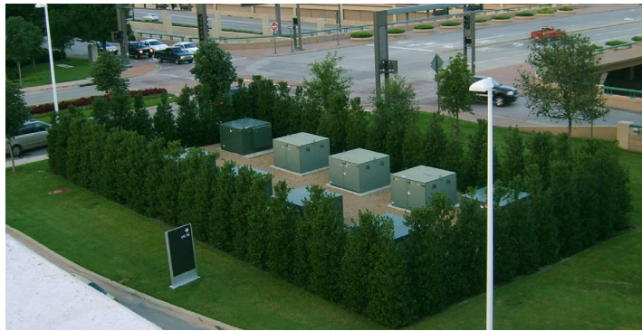
Figure 4.07.6. Example of Screened Ground-Mounted Utility Equipment
