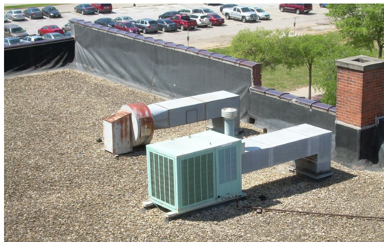
Figure 4.07.5. Example of Screened Rooftop Equipment
