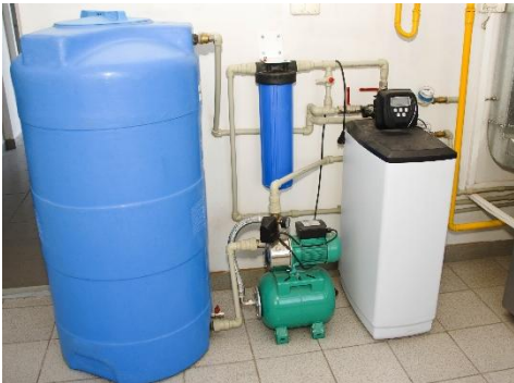
Full home water softening system
