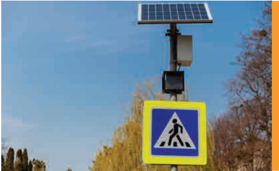
Example of Pedestrian Crossing with Retroreflective Backplate
