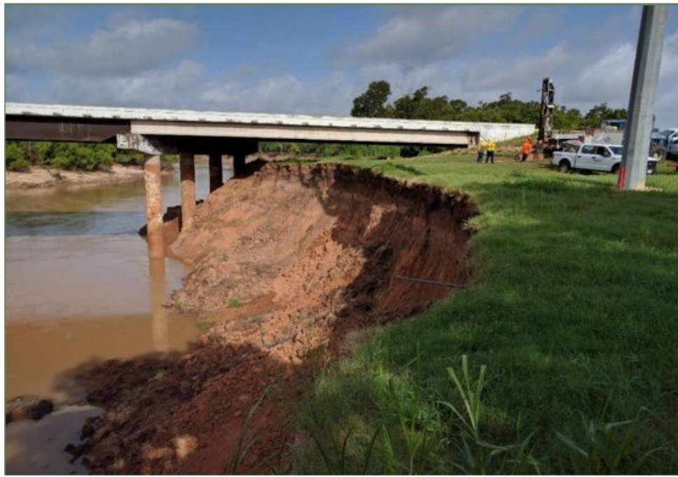
Plan form changes cause erosion at bridges, homes, pipelines
