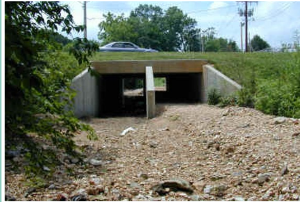
Over widened channel design results in sediment deposition
