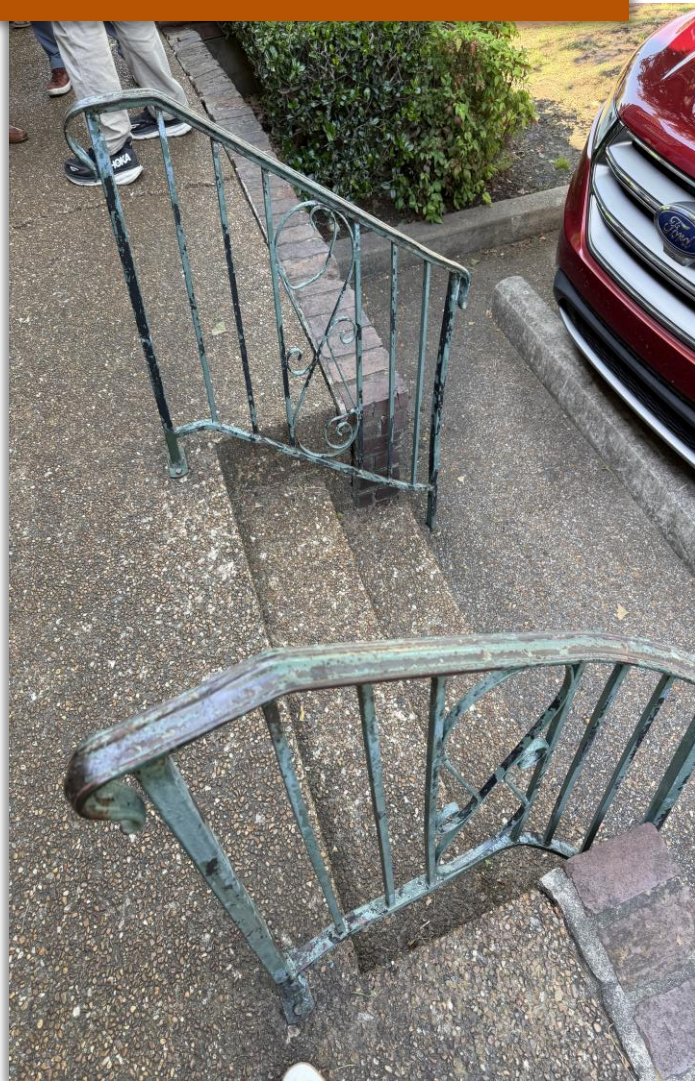
Inconsistent streetscape amenities/infrastructure
