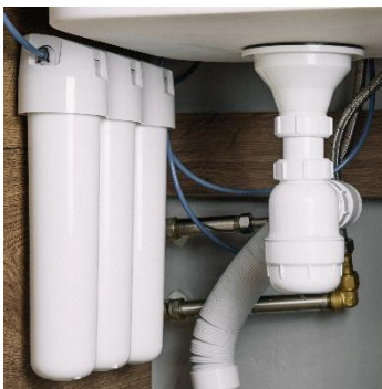
Under-sink water filter
